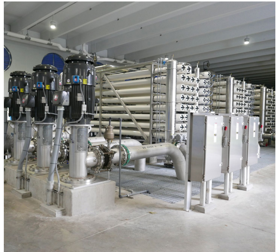
Potable water plant
