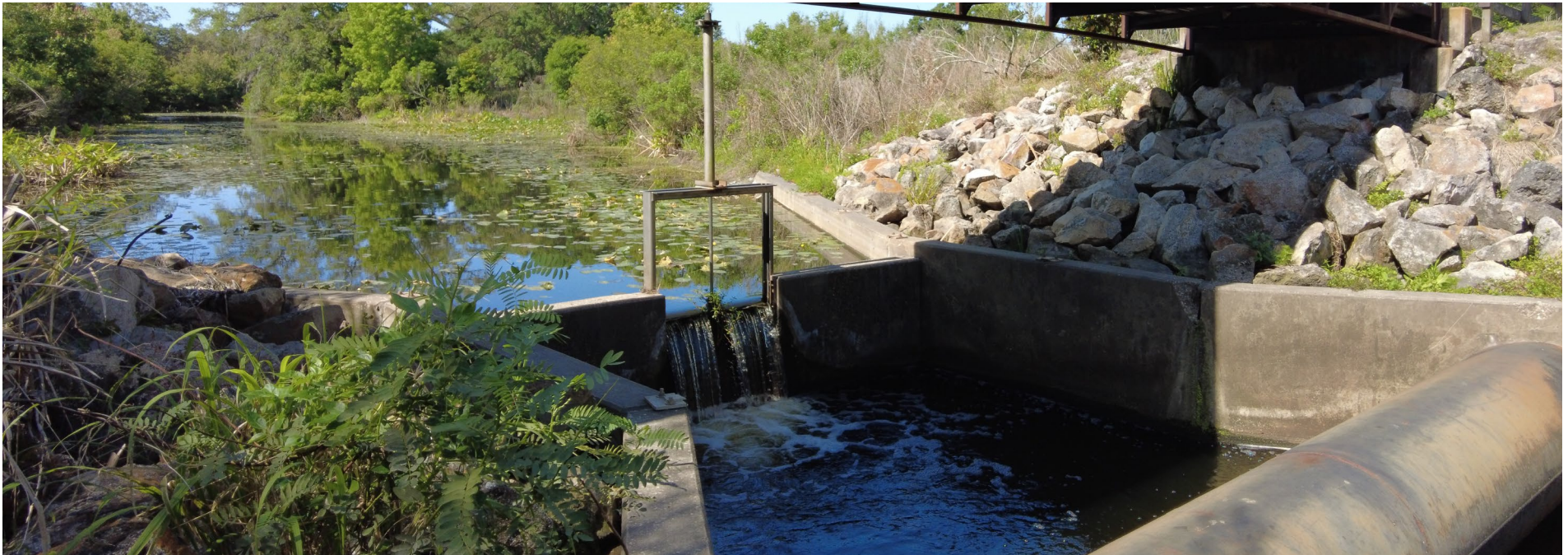
Stormwater management system in Kapok Park
