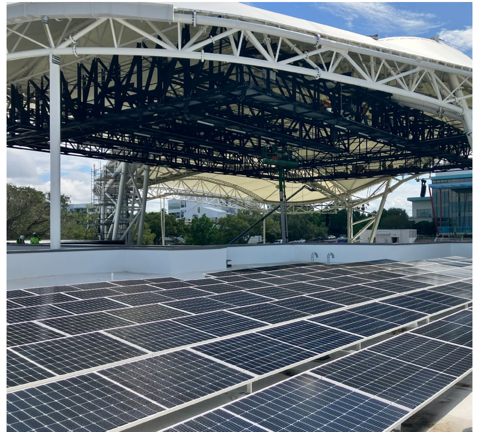
Solar installation on The Sound
