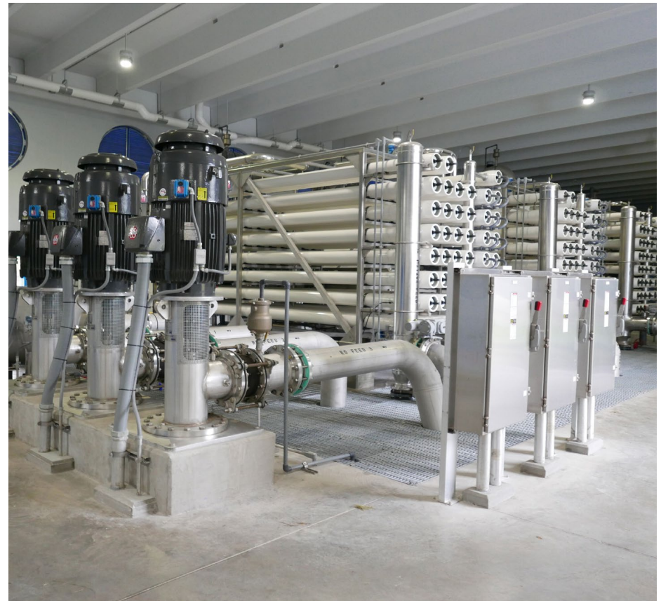
Potable water plant
